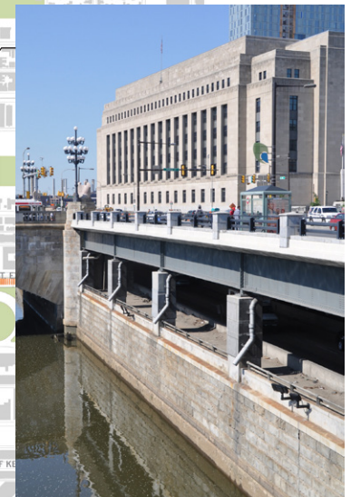
VIEW OF THE EXPRESSWAY BELOW AND SCHUYLKILL AVE. ENTRANCE RAMP ABOVE, LOOKING SOUTH FROM JFK BLVD. Credit: Parsons Brinckerhoff
